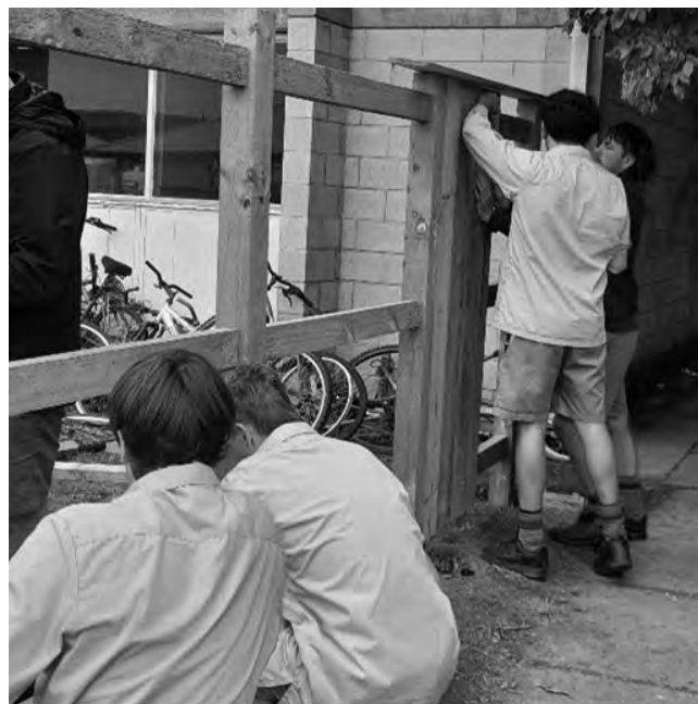
(Pictured): Commencing the first stages of the fence building, on site at College.
